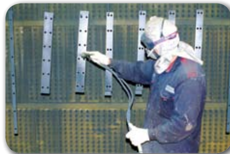
We can offer facilities of surface treatment including washing / blasting. Surface treatment is carried out with spray painting and we can even offer water based paints.
